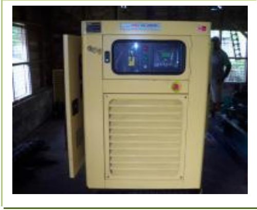
Photo 4: Karkar High School 65kVA Cummins genset
