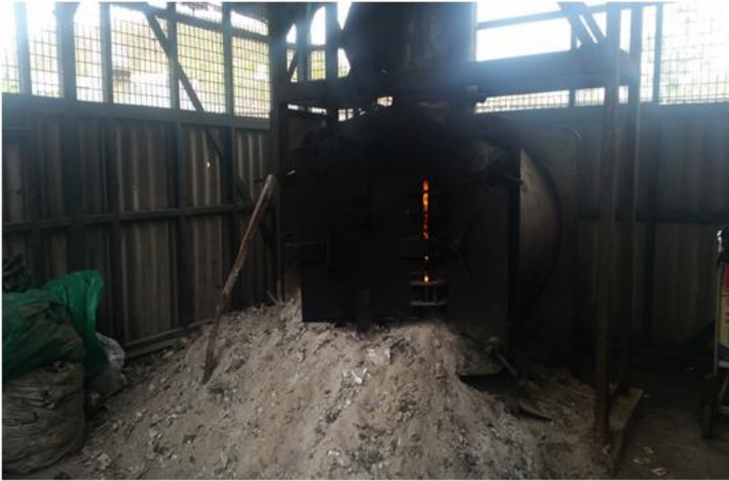
Figure 12: Incinerator at the Jackson's International Airport, PoM
