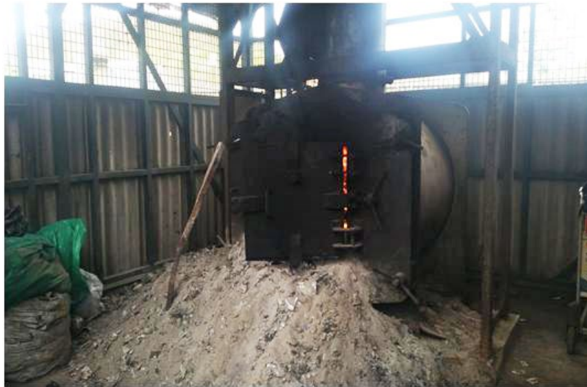
Figure 12: Incinerator at the Jackson's International Airport, PoM
