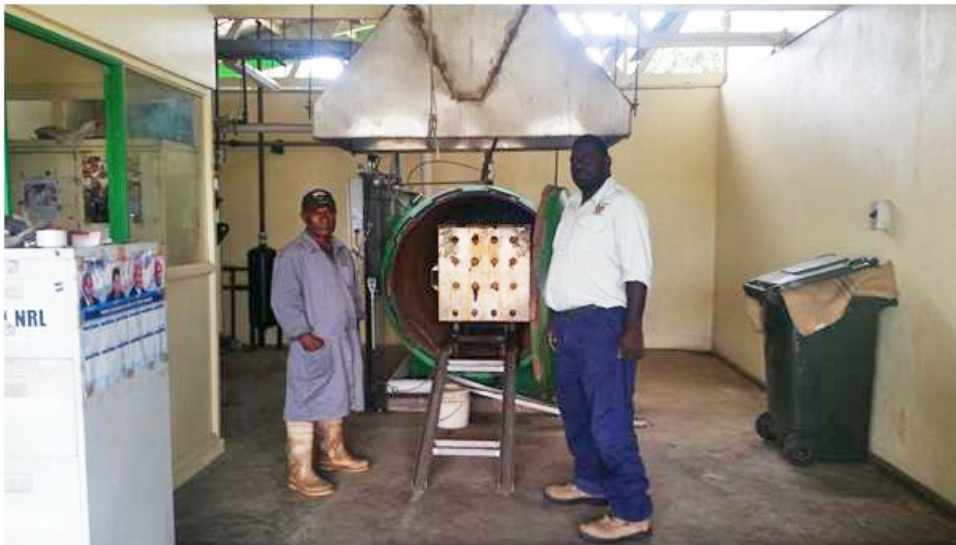
Figure 14: Inside view of the NAQIA sterilizer at the Jackson's International Airport, PoM
