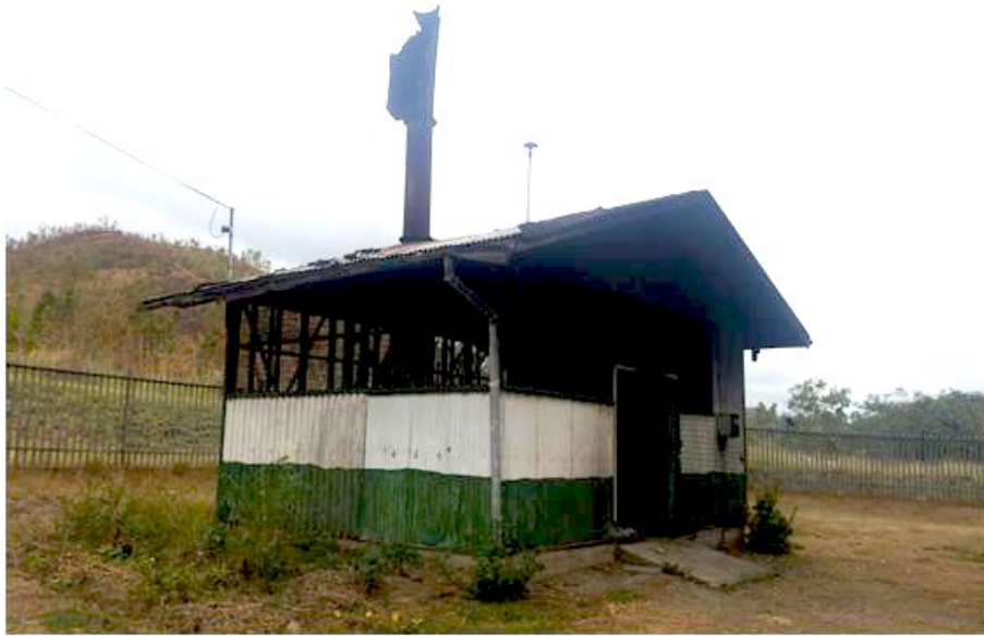
Figure 10: NW view of NAQIA incinerator at the Jackson's International Airport, PoM
