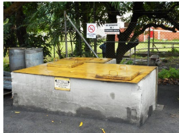
Figure 3b: Oil and water separation at Fletcher Steel
