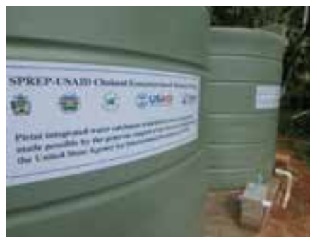
Pirini water tanks installed at the base of the catchment. Photo F.Patison/SPREP
