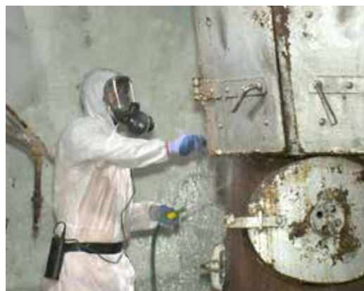
Asbestos disposal experts rid the Tamavua Twomey hospital boiler of asbestos. Photo: Amol Lal
