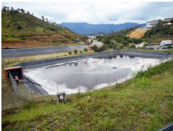
Figure 6c: CSP landfill treatment plant
