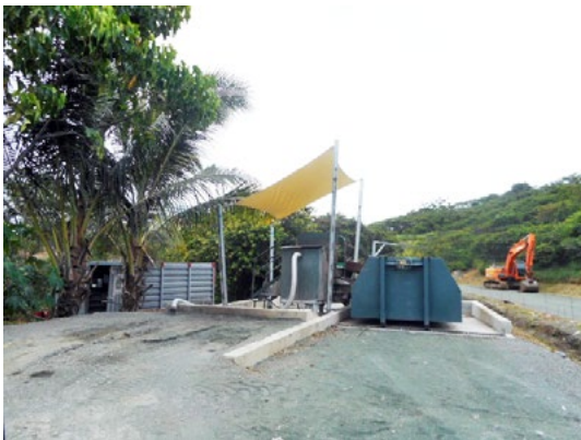
Figure 5a: Truck discharge point to sewage treatment system at CSP transfer station
