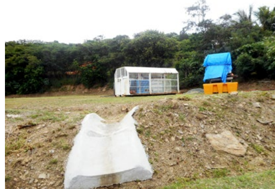
Figure 5b: Sewage treatment system at CSP transfer station
