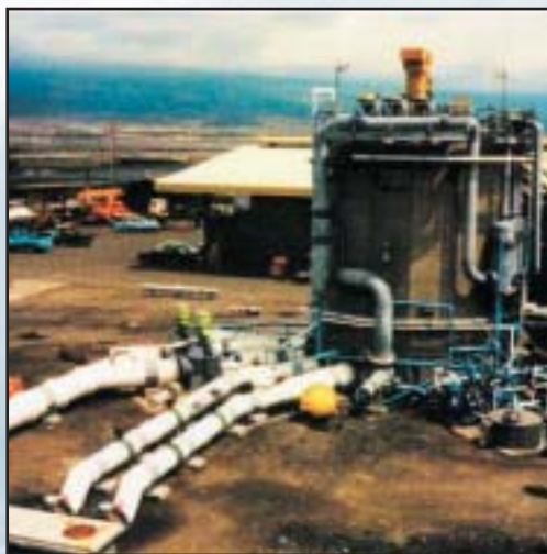
Open Cycle Ocean Thermal Energy Conservation (OC-OTEC) system located at the Natural Energy Laboratory of Hawaii Authority (NELHA) at Keahole Point on the Big island of Hawaii.
