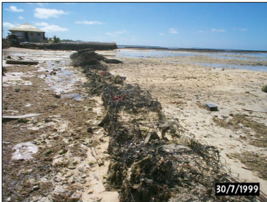
Figure 8.8. Scouring alongside a gabion basket seawall in south Tarawa, Kiribati.
