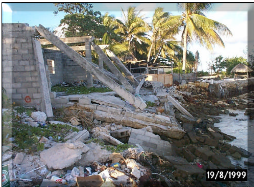
Figure 5.5. Failure of shorefront buildings due to wave action, Tarawa, Kiribati.
