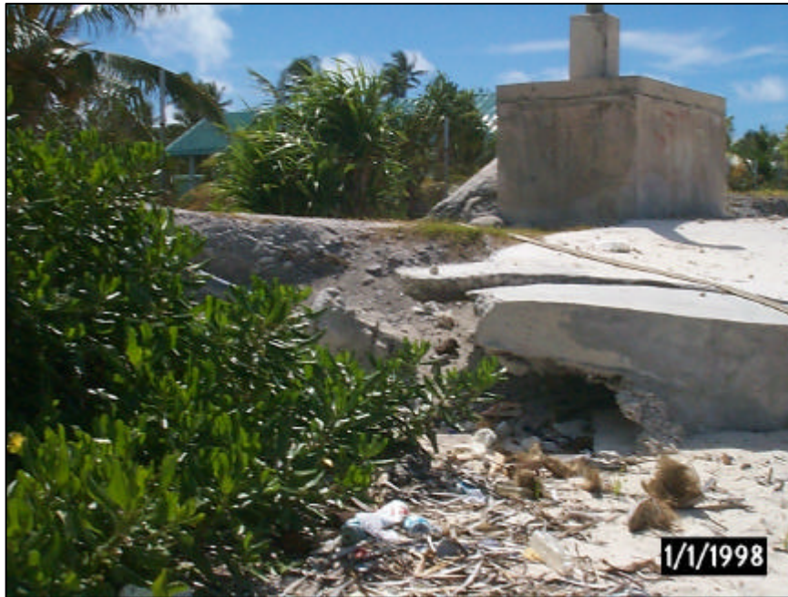
Figure 8.7. Collapse of a shorefront building due to foundation scouring in Tarawa, Kiribati.
