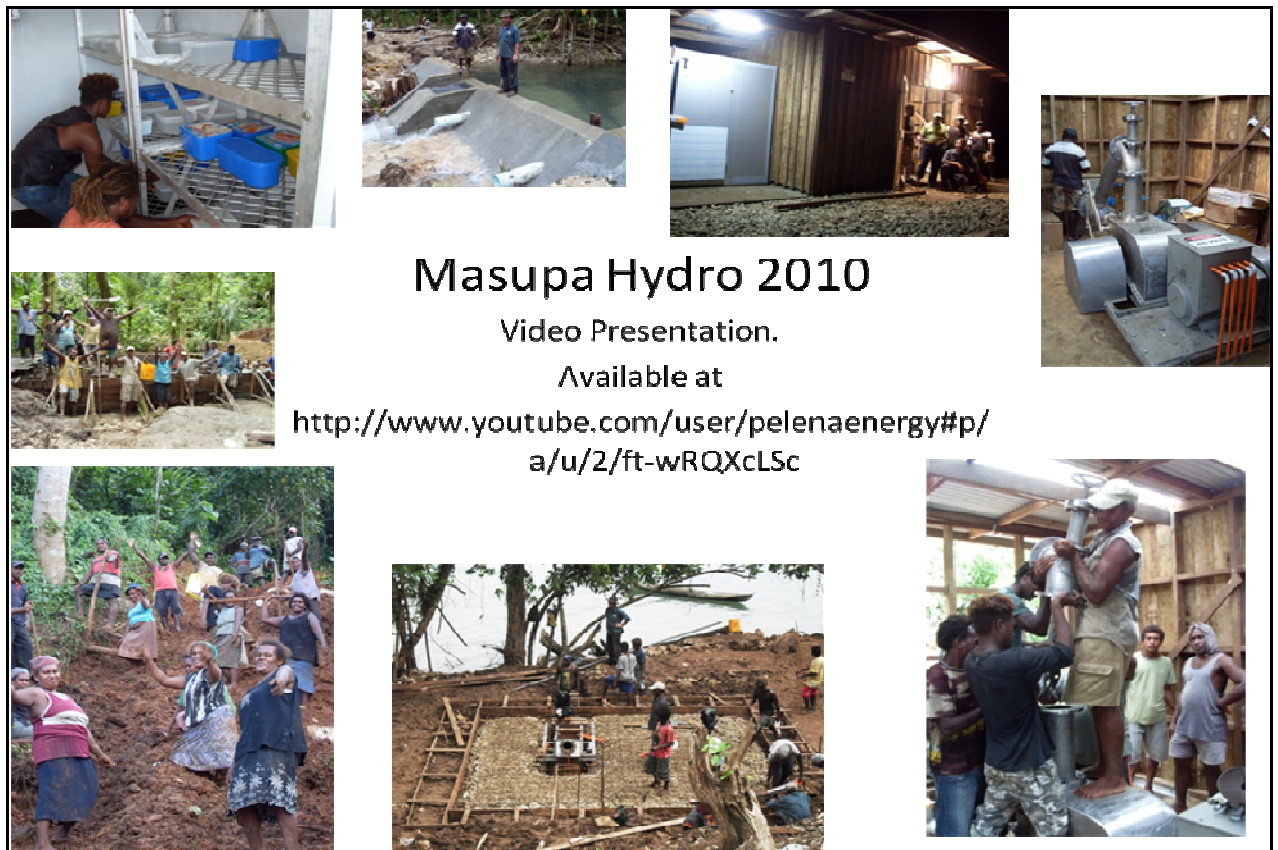
Figure 4: Various photos from the 13-day construction of the Masupa Hydro in Jan/Feb 2010.
