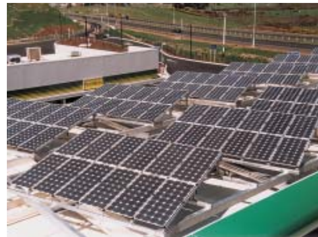
Solar Panels provide electricity for this BP service station Bruce Jarvis
