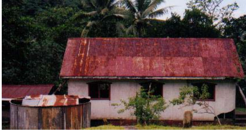
Fig: 11. Corrosion of roof catchment from salt spray and volcano induced acidic rain
