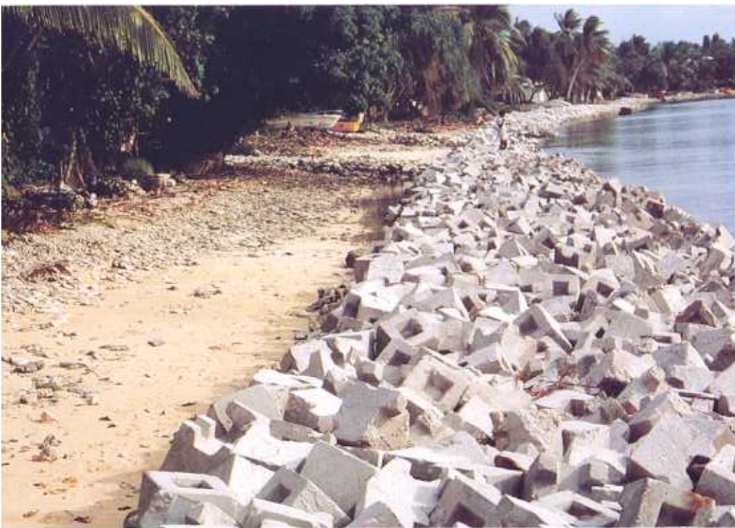
Plate 32. Small concrete cubes placed randomly to form an extensive length of coastal protection along the lagoon beach of Fongafale, Funafuti Atoll, Tuvalu.
