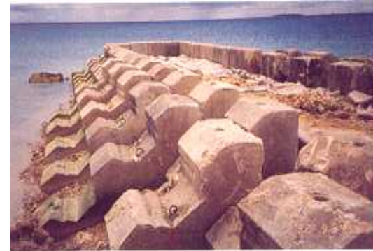
Plates 39 and 40. Heavy concrete armouring units being constructed on site, and put in place as an artificial breakwater at the Naval Base in Nuku'alofa, Tonga.
