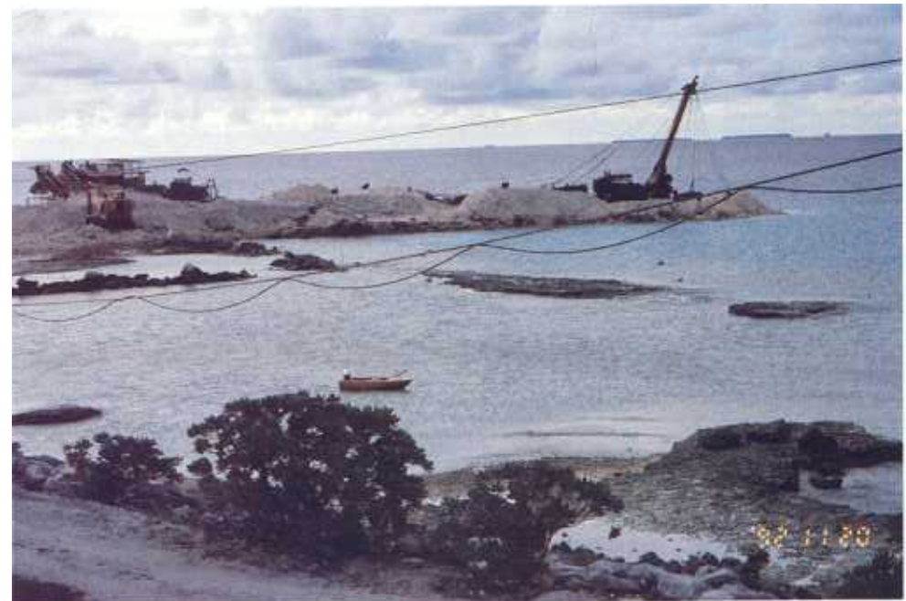
Page 20. Dredging for sand using a dragline on the lagoon side of Majuro Atoll, Marshall Islands.
