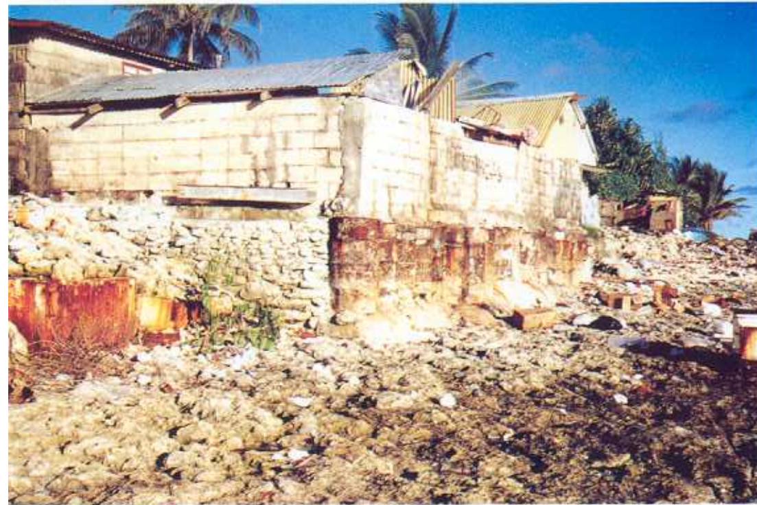
Plate 21. Vertical concrete block seawall and 44 gallon drums full of concrete protecting property on the ocean side reef flat of Majuro Atoll, Marshall Islands.
