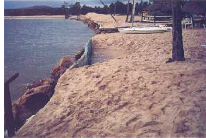
Plate 16. A beach forming part of a sand spit being eroded and threatening buildings at the Shangri-La Fijian Resort in Fiji. Note that attempts at protection using pine pole logs and large coral blocks do not appear to have been successful.
