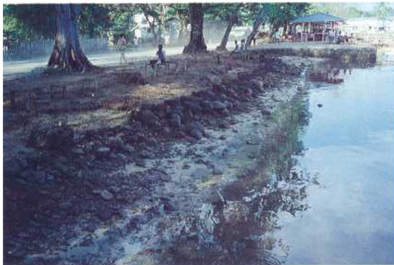
Plate 30. Erosion of the narrow beach threatening the road and water front area of Gizo, New Georgia, Solomon Islands. Note the attempts at protection which include a rubble rock wall in front of the road and gabion baskets around the market stalls in the distance.
