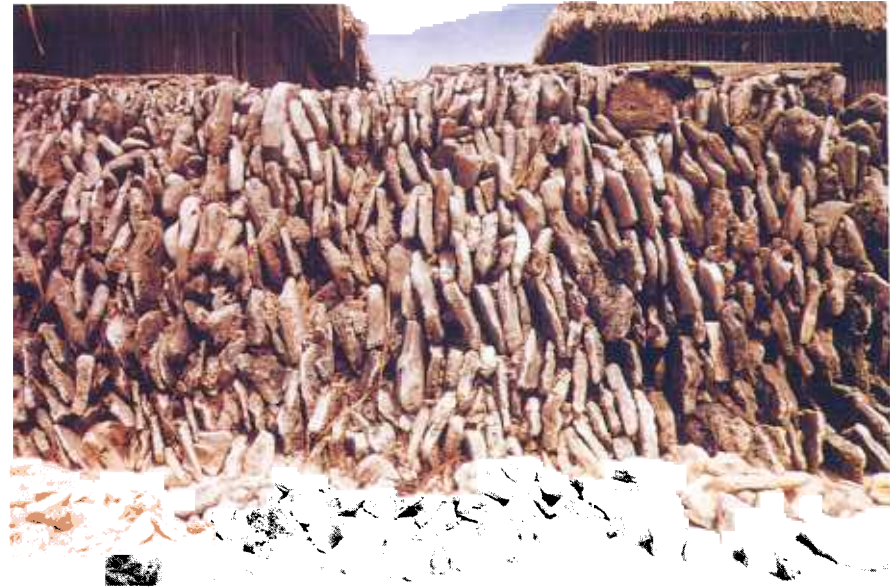
Plate 36. A near-vertical seawall of coral and beachrock slabs stacked over 2 metres high.
