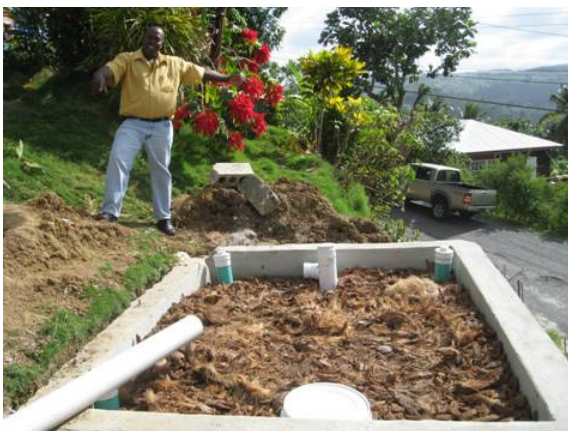
Accessible technology solutions, such as this wetlands filtration system, are being constructed in Saint Lucia as part of an overall approach to managing wastewater in a changing climate. (Photo by Donna Spencer).
