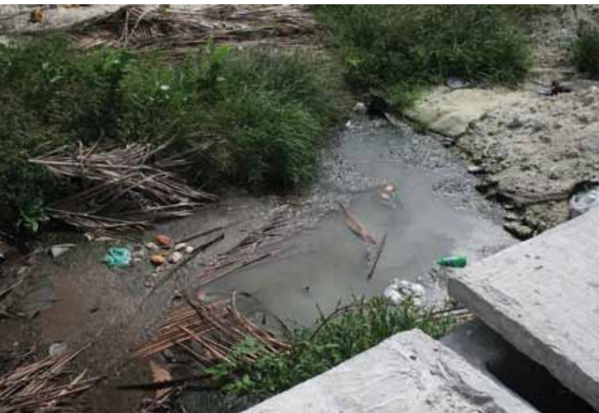
Drainage channel on Viligili with water logging
