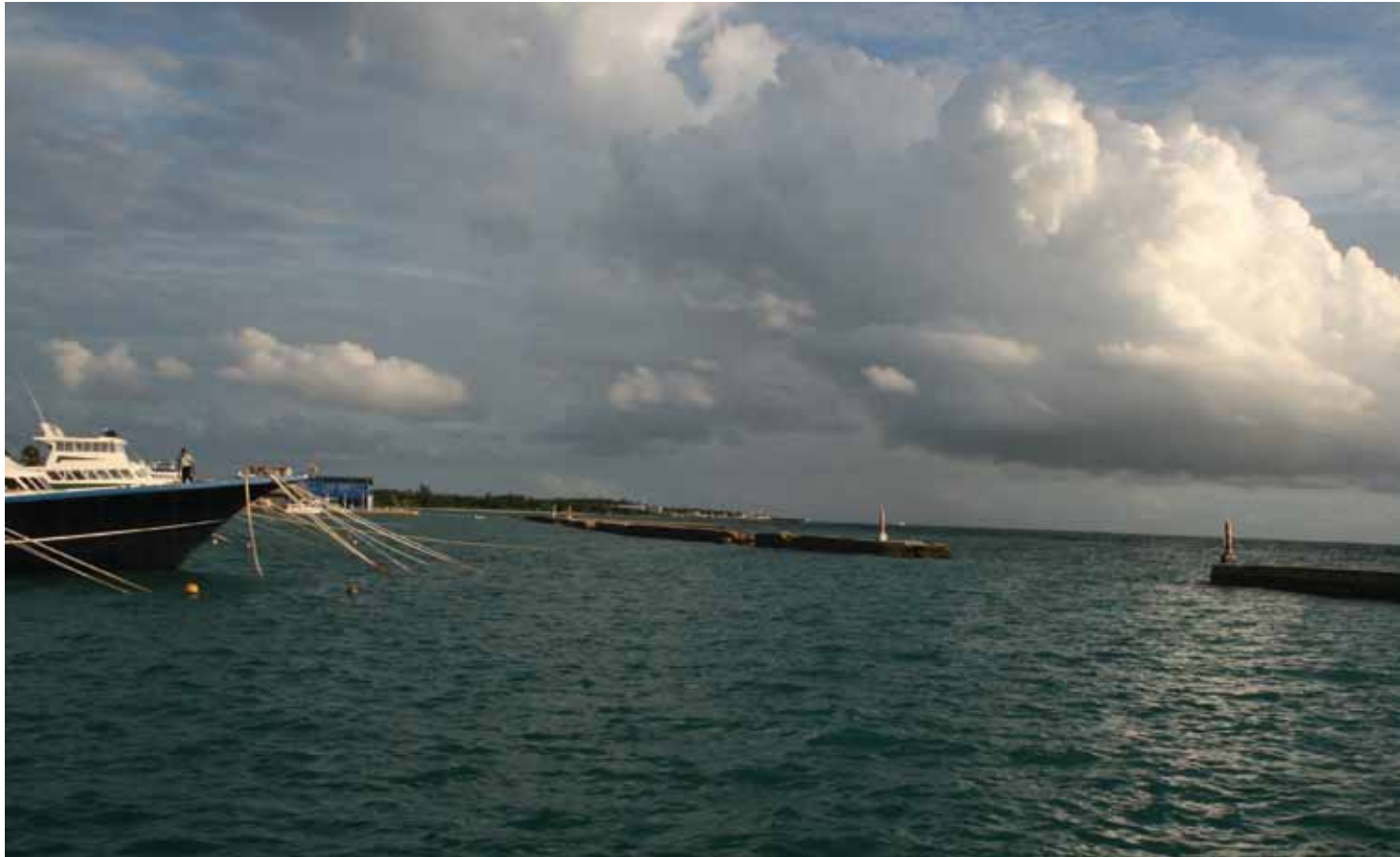
Viligili harbour wall and entrance facing the prevailing weather and showing clear signs of wave damage that occurred in January 2008
