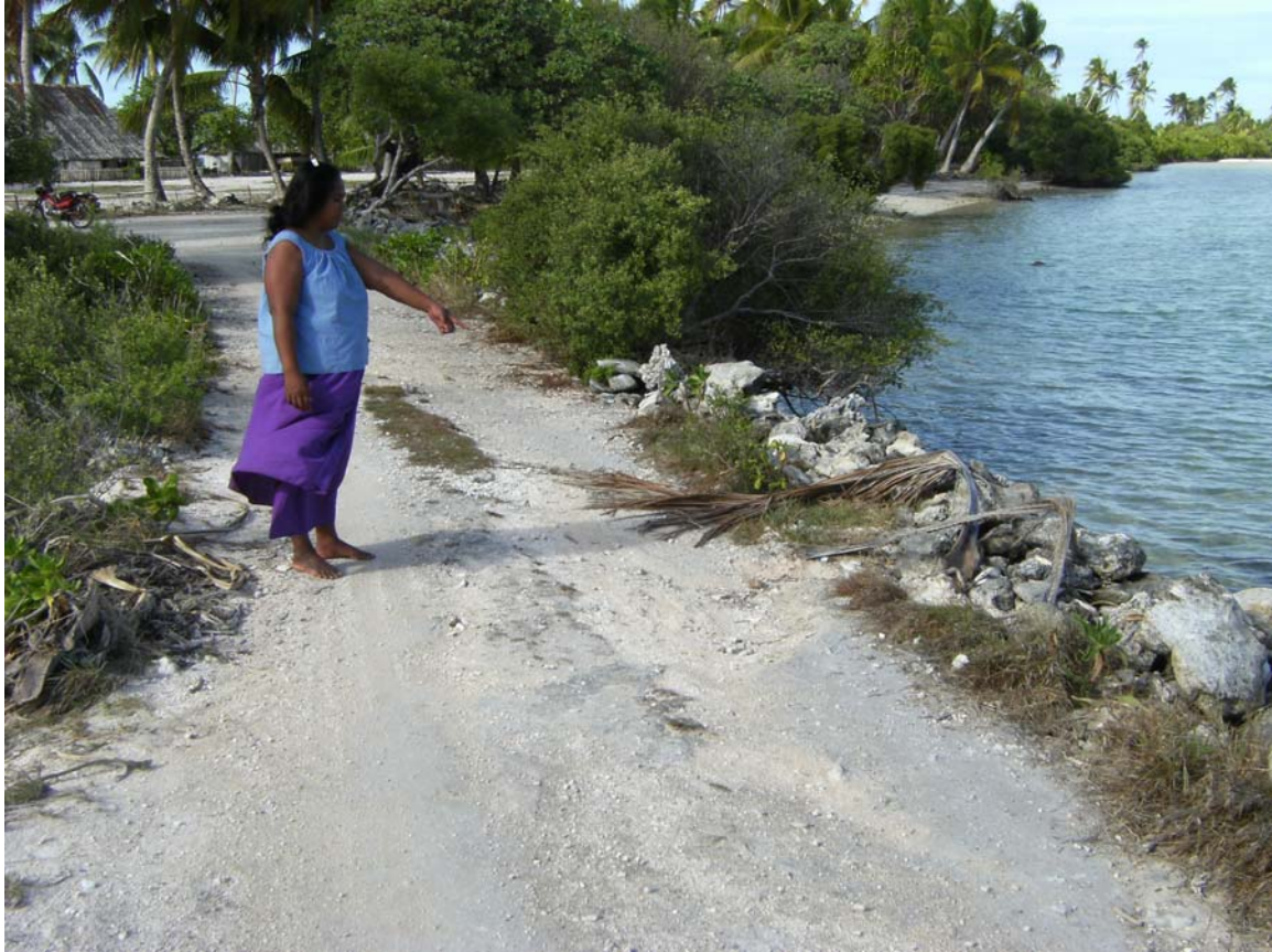
Figure 8. Eroding shoreline and seawall, Butaritari, Kiribati
