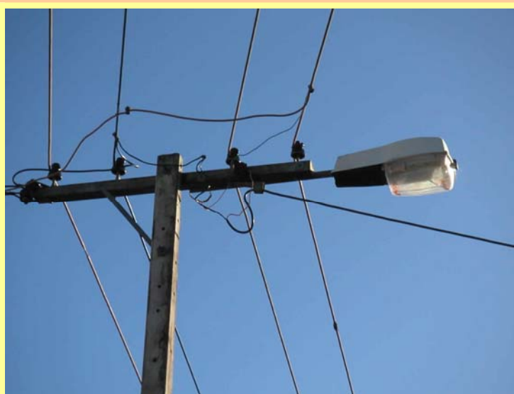
Picture 3-11 Street Light
