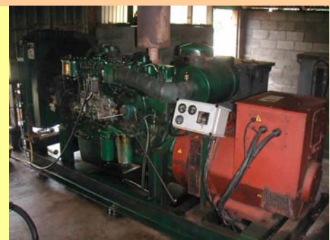
Picture 3-10 Hino Generator
