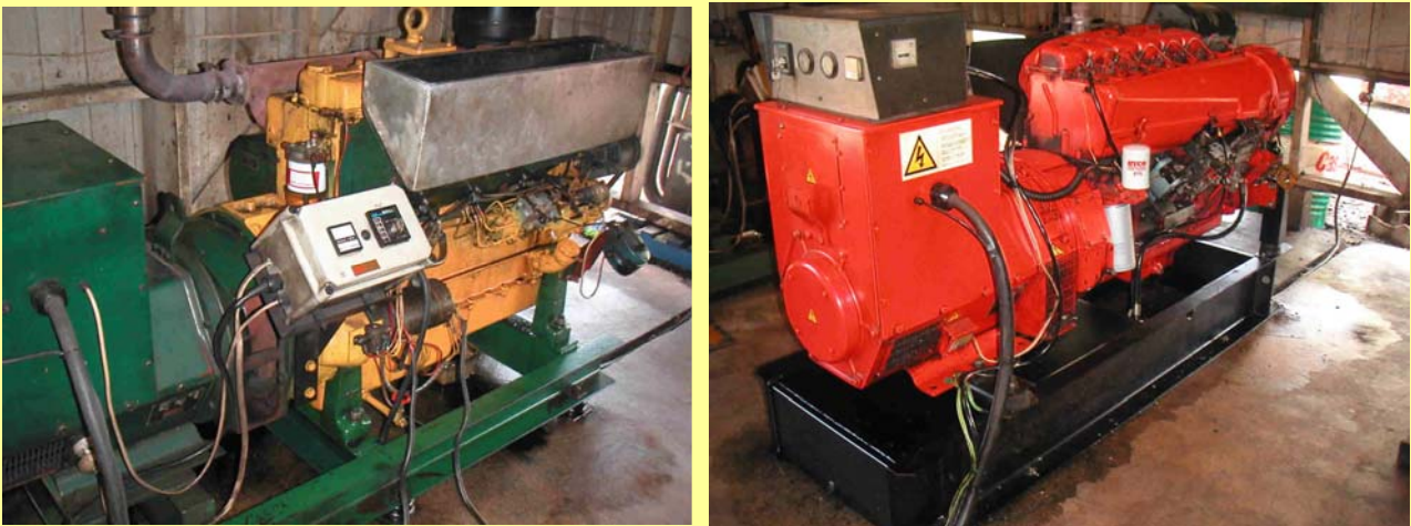
Picture 3-9 Lister and Deutz Generators
