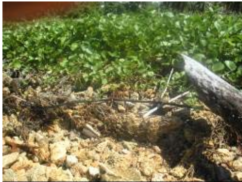
Photo 5-8 Broken shore protection with broken wires
