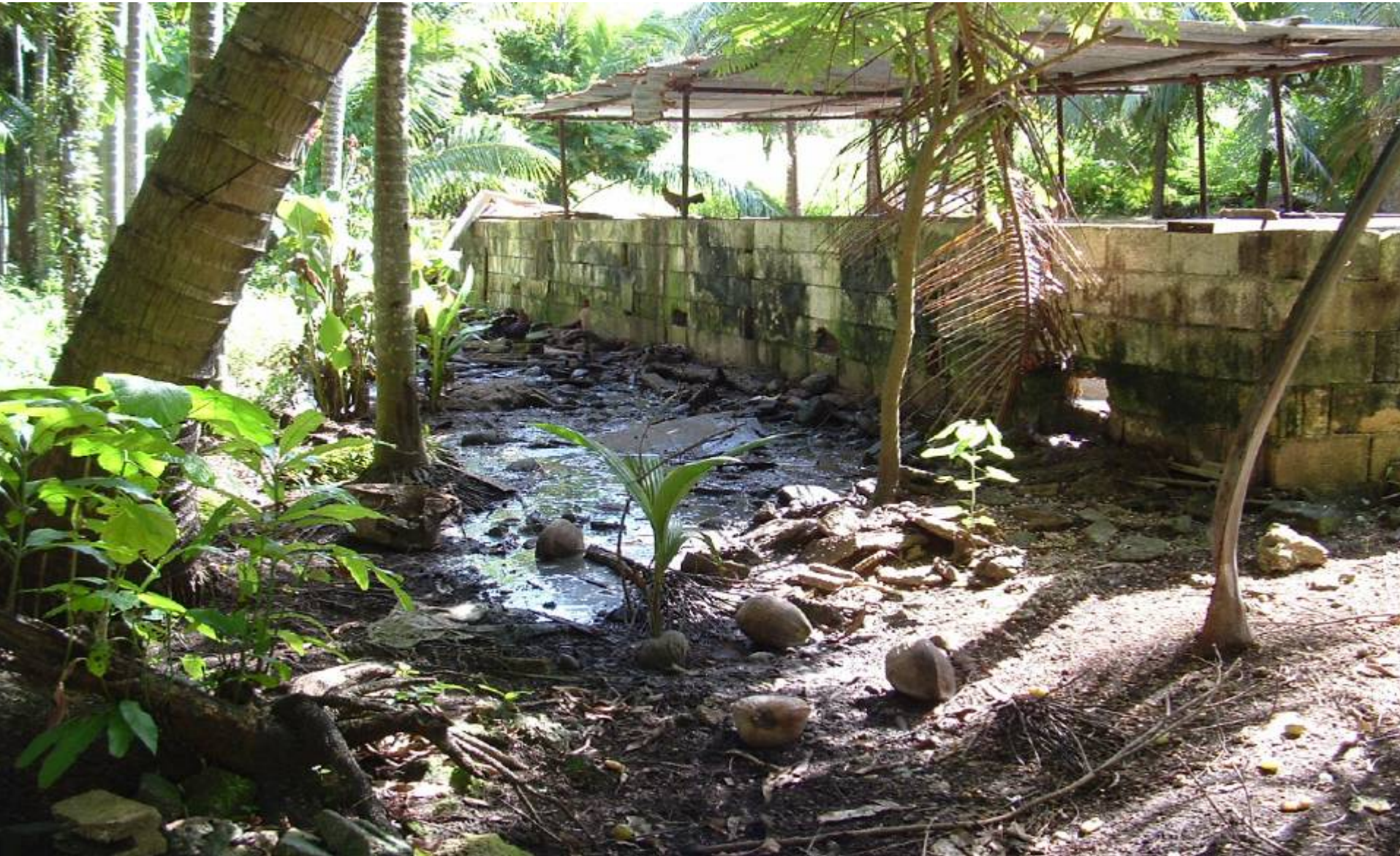
Uncontrolled flow of manure around the perimeter of the piggery (Tinian)
