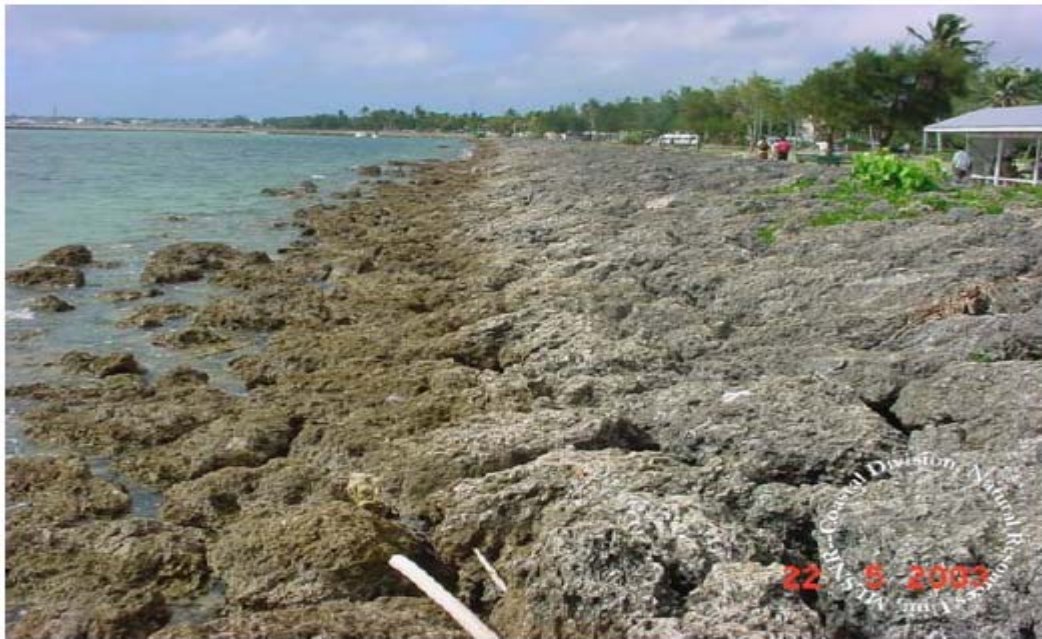
Figure 2.18: Coastal Foreshore Protection Wall at Nukuálofa Waterfront Source: Ministry of Lands, Survey & Natural Resources, 2003.
