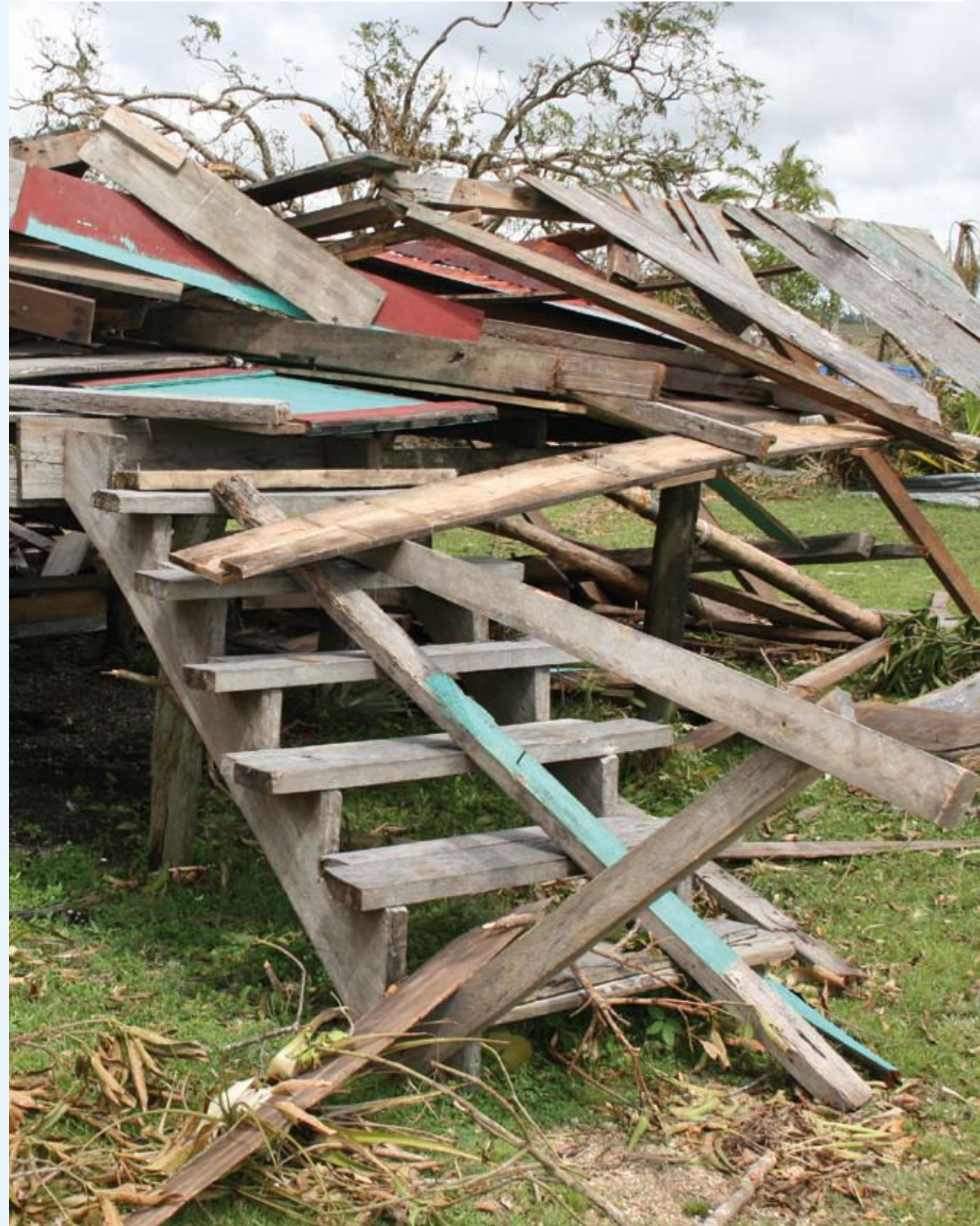
Damage by Hurricane Felix in Krukira, Nicaragua. Virtually everything built of wood collapsed. The few buildings left intact were concrete. Photo: Alex Wynter/International Federation of Red Cross and Red Crescent Societies
