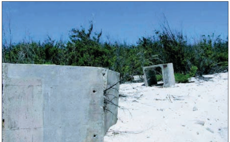
Figure 11.11 Concrete blocks filled with sand and coral rubble to form a seawall were carried tens of meters up the beach on Wake Island. Photo: J. Miller.
