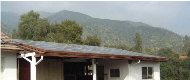
Figure 8. Direct Grid Connected Fixed Solar Panels, 5 KW system. Note that solar panels are only on one half of the roof (i.e. what is shown in image).
