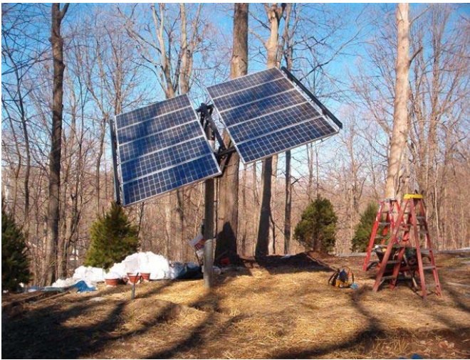
Figure 7. Direct Grid Connected Two-Axis Tracking Solar Panels, 1.2 KW system.
