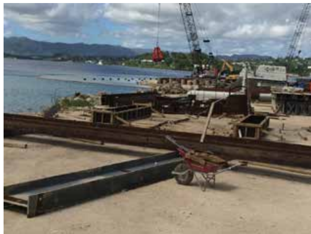
Reconstruction and upgrade of Lapetasi Wharf at Port Vila, Vanuatu with funding from DFAT (feasibility study) and JICA (construction works), Vanuatu Project Management Unit
