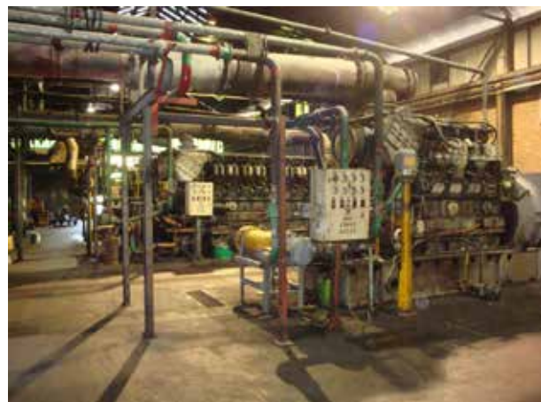
Power plant at Nauru Utilities Corporation (J. Overbeek)
