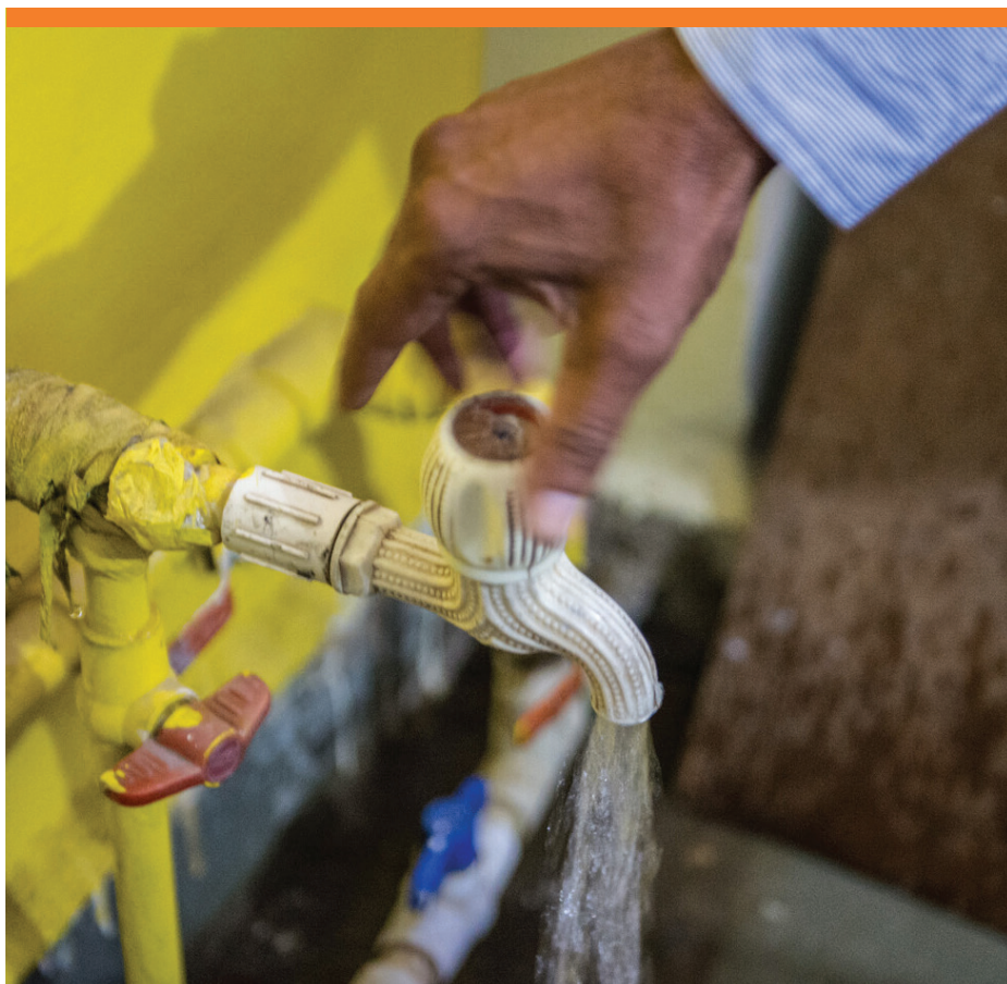
Leaky pipes. Nonrevenue water creates a loss of about 40%-50% (photo by Ariel Javellana/ADB).
