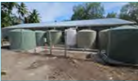
New rainwater harvesting system at Polowat Elementary School, Polowat Island, Chuuk State, FSM
