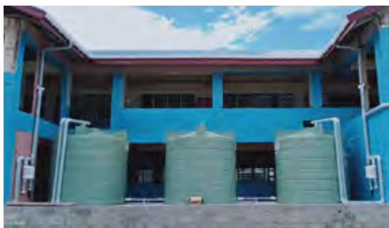
Rainwater harvesting system at Fetuvalu Secondary School, Funafuti, Tuvalu
