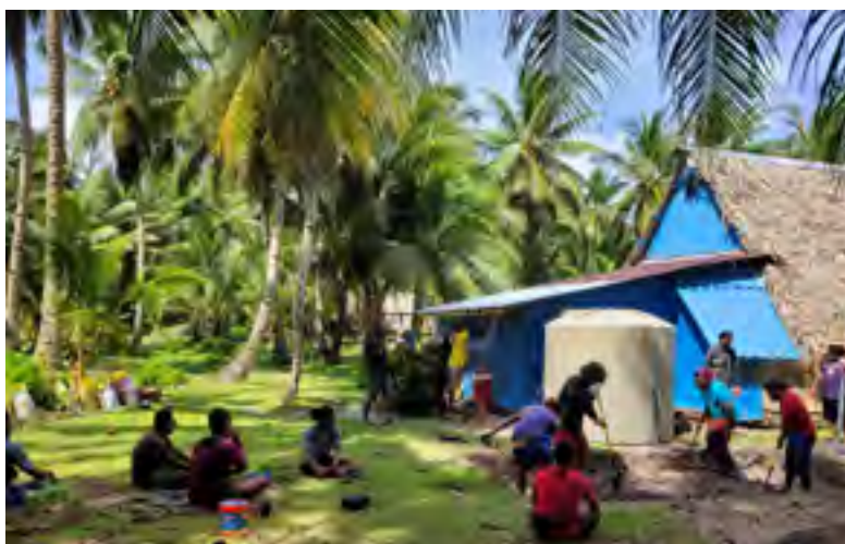
Community members assisting with the installation of a rainwater harvesting system at the Catholic Church, Pulusuk Island, Chuuk State, FSM
