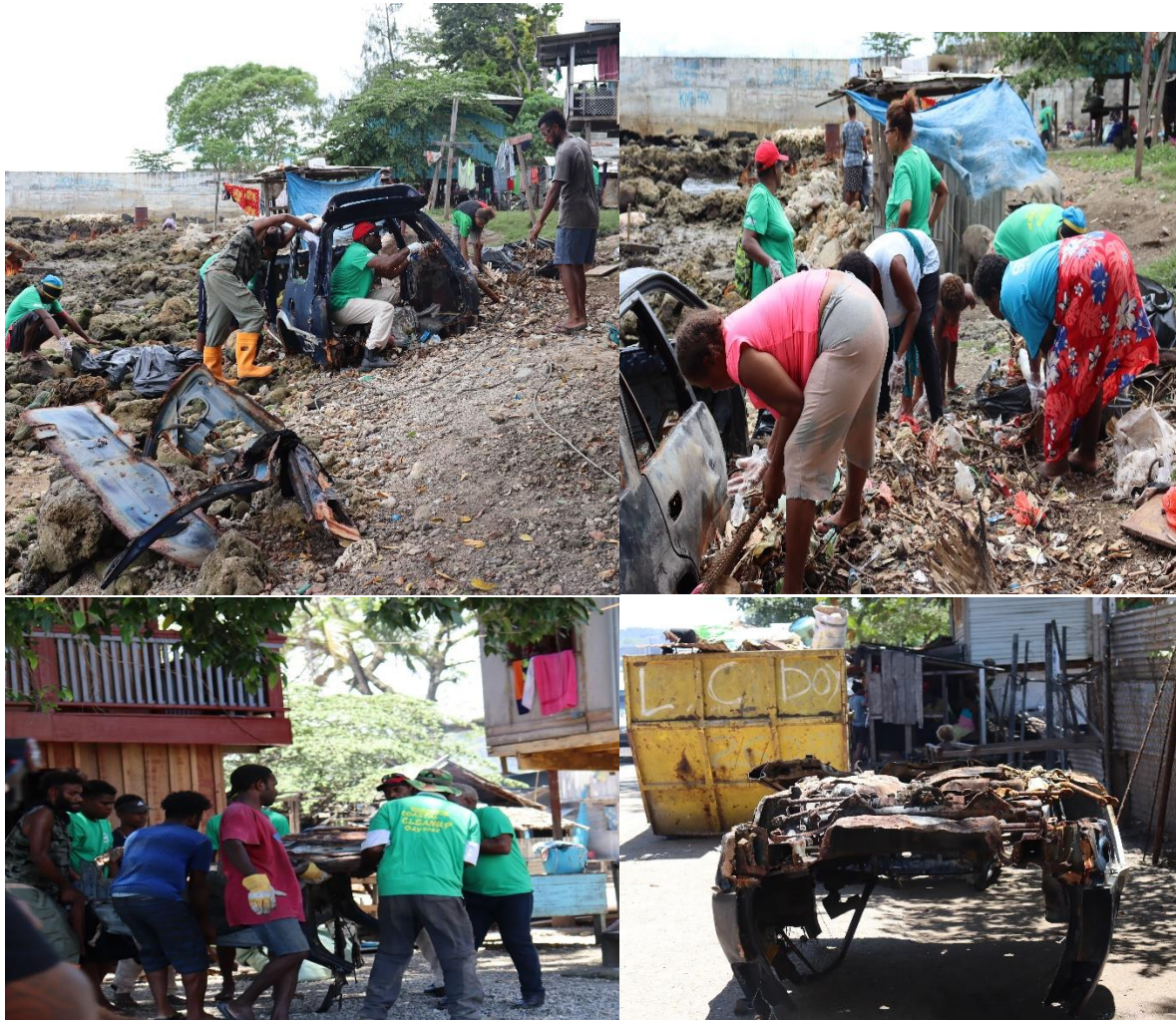
Fig.10. Removal of Bulky wastes using Electric grinder and other heavy wastes to yellow Skip Bin storage site
