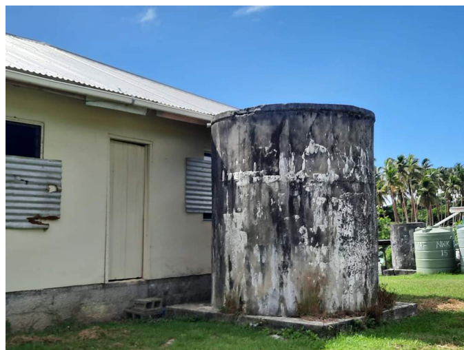
Household water tank in Nacula village.
