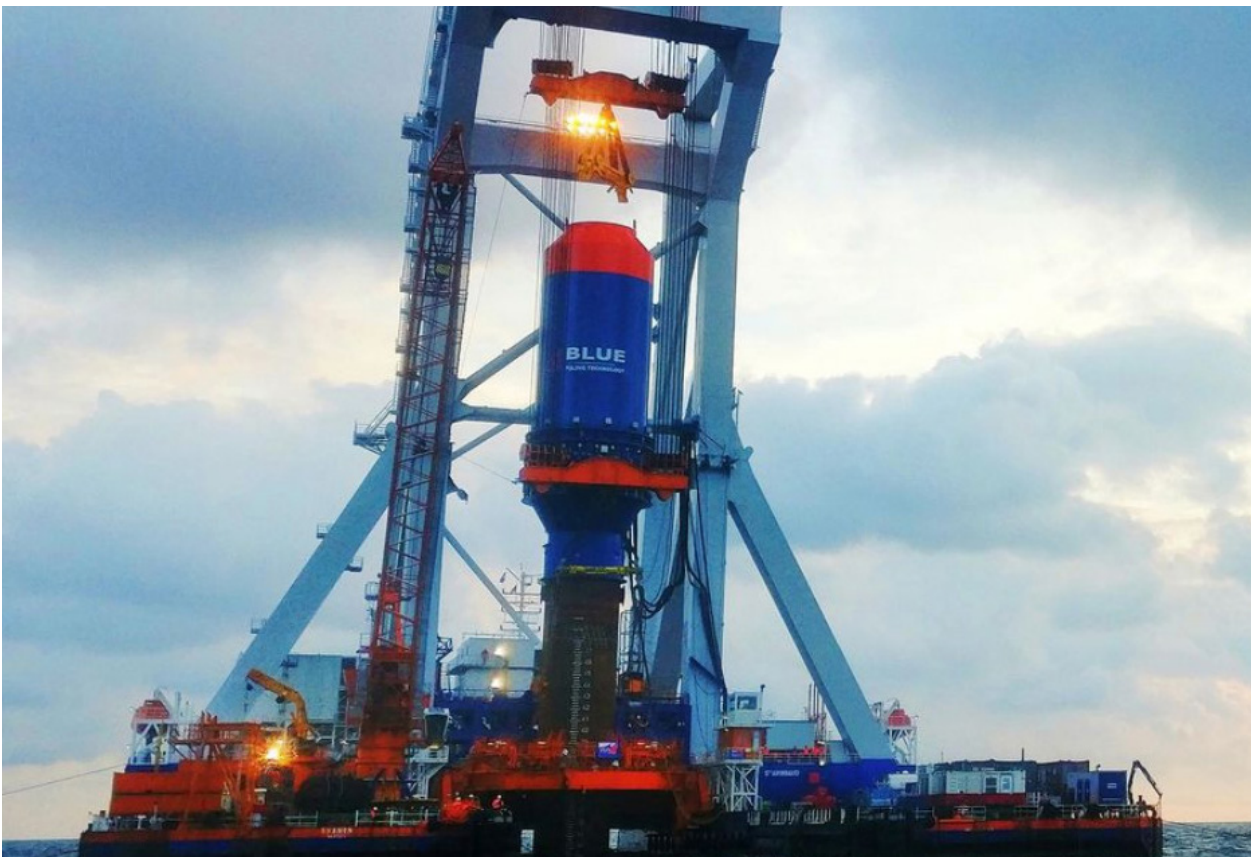
Picture 9. BLUE Piling is a new technology being tested and employed to reduce both underwater noise and material fatigue. © iqip.com
