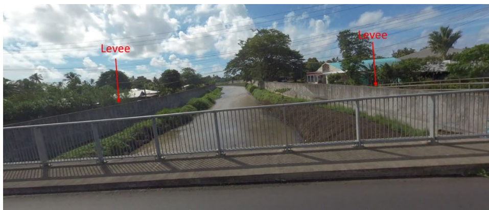
Figure 56. Levees in the Vaisigano river at the Faatoia Bridge. Figure taken from Google Maps.
