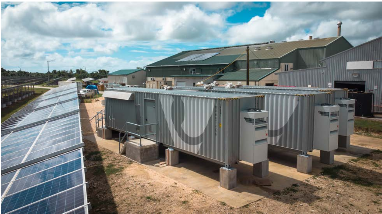
Popua Power Station, Tongatapu, Tonga. An example of a large-scale project (photo by TPL).
