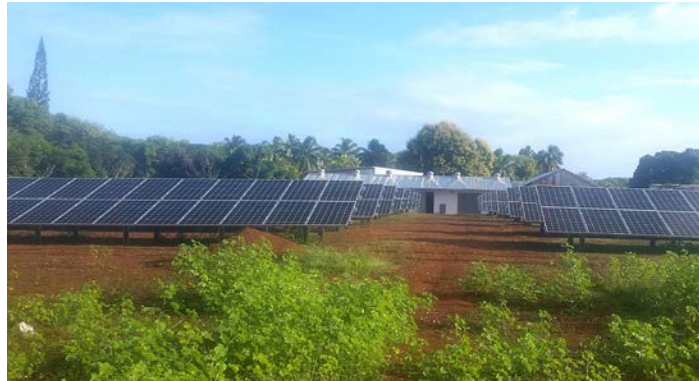
Mauke Hybrid Power Station in the Cook Islands. An example of a small-scale project (photo by Entura).
