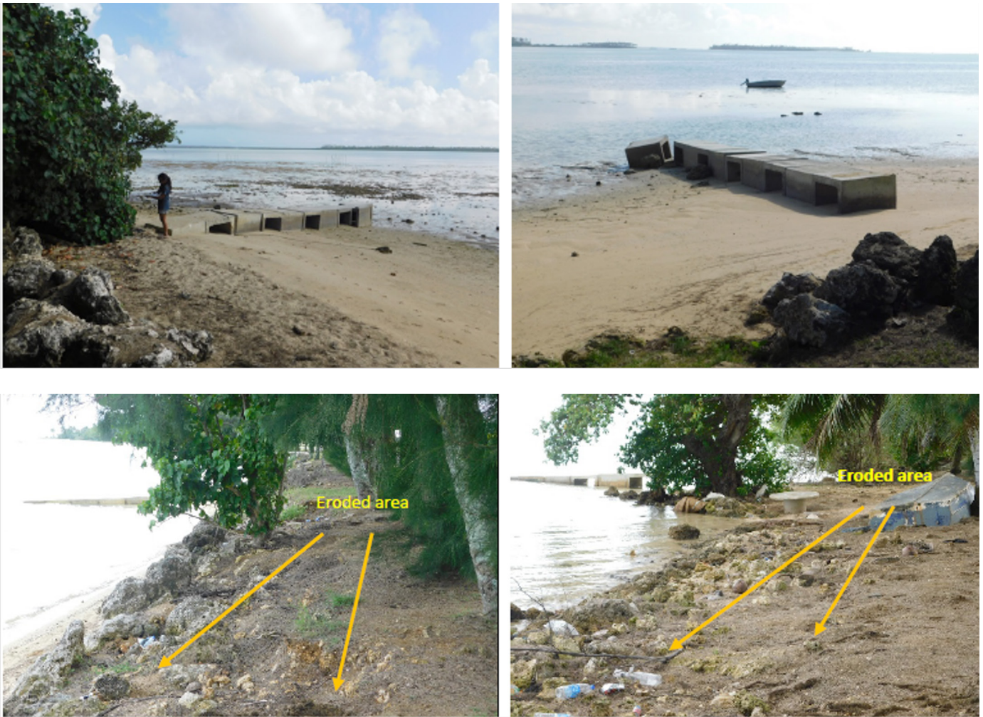
Figure 7. Photographs (top two) groyne structure showing sand accumulation at 50% permeability. (bottom) photographs show signs of erosion near groynes #11 and #12. Hahake along Makauga-Talafo’ou coastlines. July 2021.
