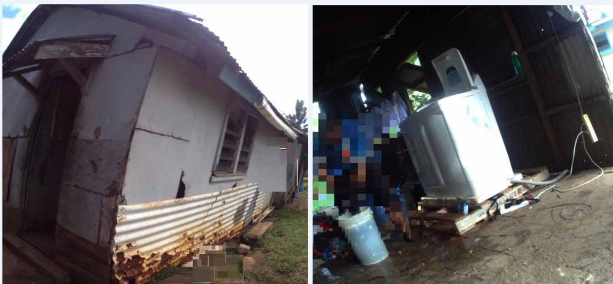
Images from the Tongatapu housing and health study. Left: Poor building quality indicated by holes in the external wall and use of building materials to patch up exterior. Right: electrical extension blocks and power cables next to a washing machine and in the vicinity of a water spill.
