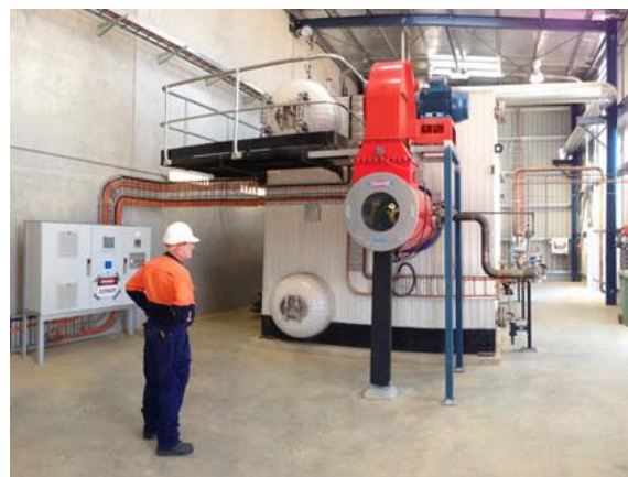
Image: steam boiler system with emission capture (Fiji)
