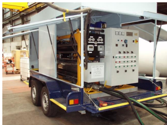
Image: trailer mounted transformer oil filtration unit (Australia)
