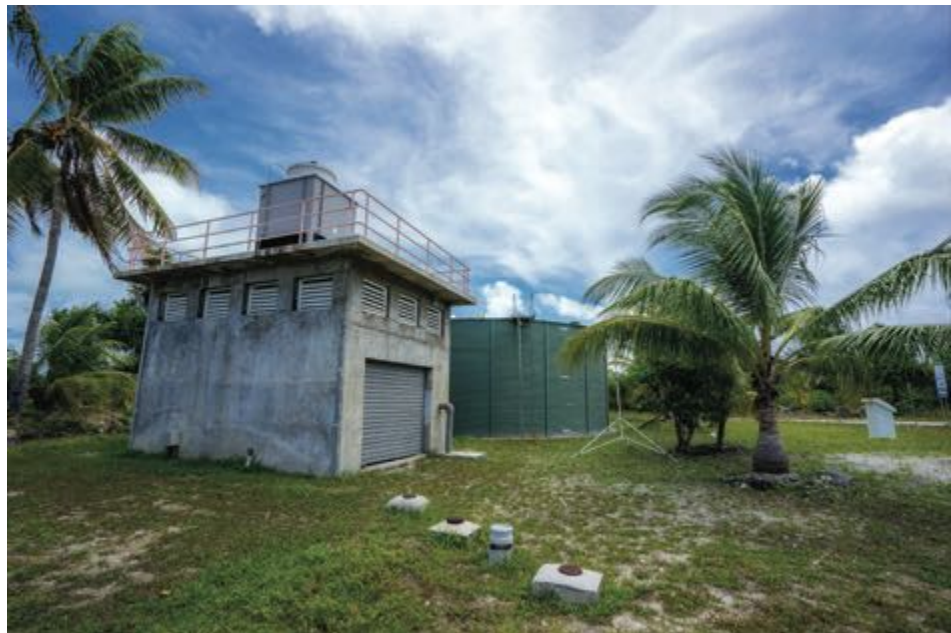
Existing aeration system for sulfur removal and water storage tank at Bonriki (photo by ADB).
