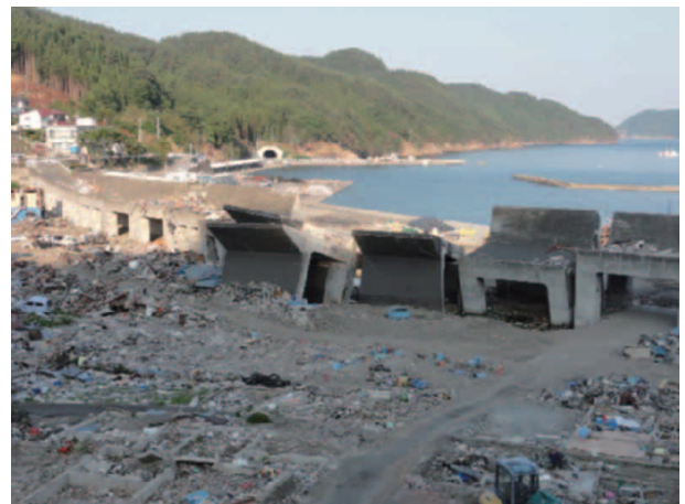
Figure 5-3-2 Damage to the coastal levee and the residential area (Touni, Kamaishi City, Iwate Prefecture)
