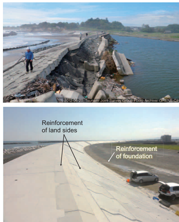
Figure 5-3-3 Top : Typical break of the coastal levee (Soma City, Fukushima Prefecture) Bottom : Restored coastal levee(Watari Town, Miyagi Prefecture)
