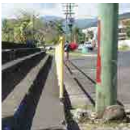
The seawall, access ways and footpaths need to be redesigned to ensure accessibility for all
