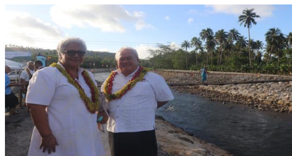
The River Protection Rock Wall at Lalomauga. Deputy Prime Minister, Fiame Naomi Mataafa carried out the ribbon cutting of the ceremony.
