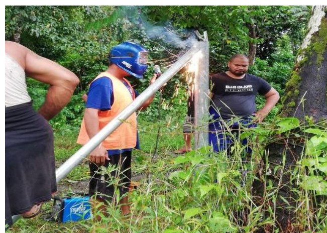
Welding of fence posts and some of the tree species planted during the tree planting with the community
