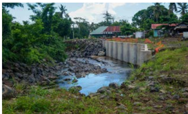
Flood protection near Malia’s home. The Green Climate Fund is supporting work to benefit 27,000 people living in the flood-prone Vaisigano river catchment in Apia, Samoa.
