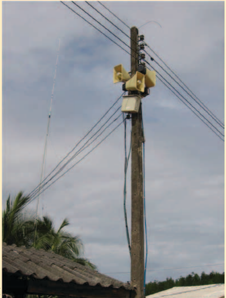
Loudspeakers installed as part of actions to strengthen community early warning systems. Thailand
