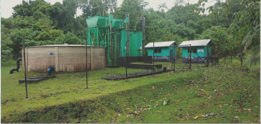
Figure 11: SWA Water Treatment Plant
