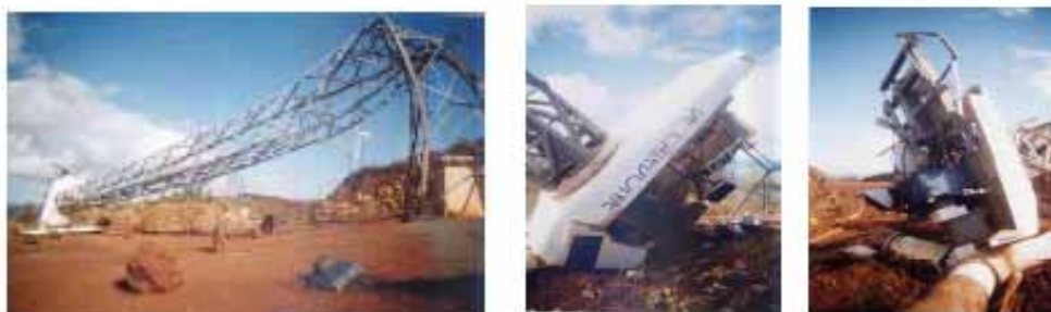
Cyclone Damage to Plum wind farm, Source: Small Wind Industry Implementation Strategy)
