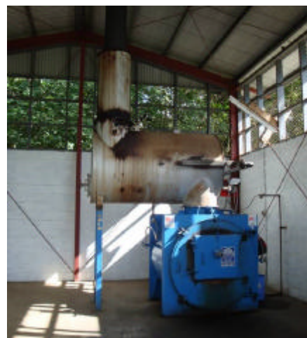
Medical Waste Incinerator in Samoa
