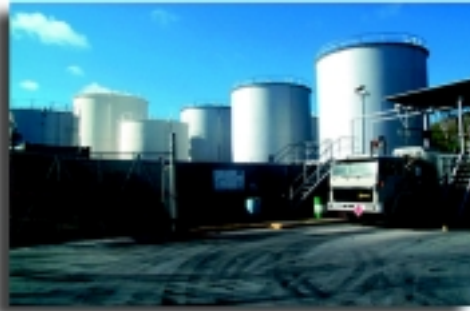
Oil storage tankers
