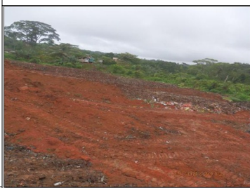
Caption : Ground Works on at Gizo progressing and Honiara is still undergoing clearance and leveling .
