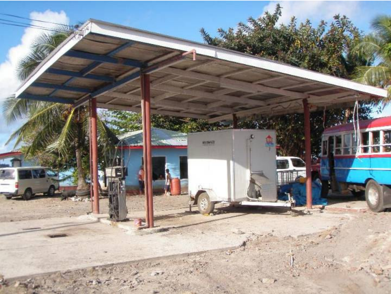
Plate 4: Damaged petrol station, Vailoa
