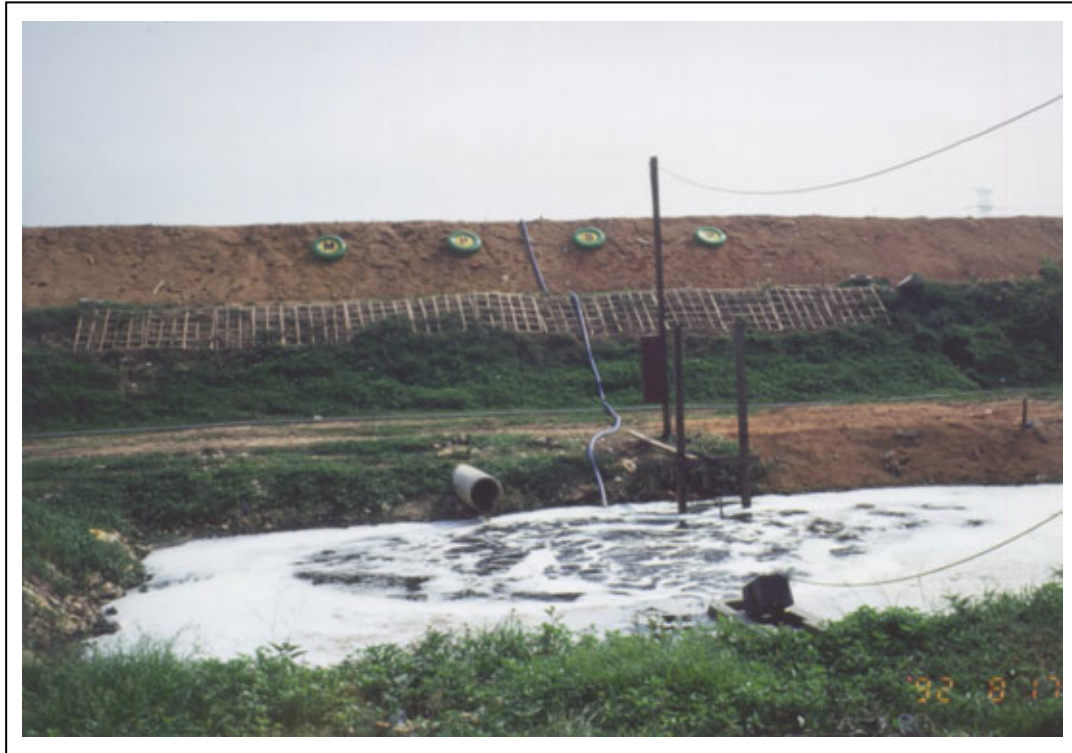
Picture 2-7 Example of leachate discharge pipe opening that is appropriately opened (leachate natural flow discharge method)
