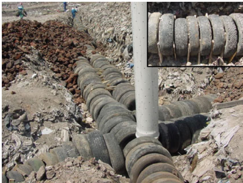
Picture 2-5 Example of using waste tires as leachate collection discharge pipes
