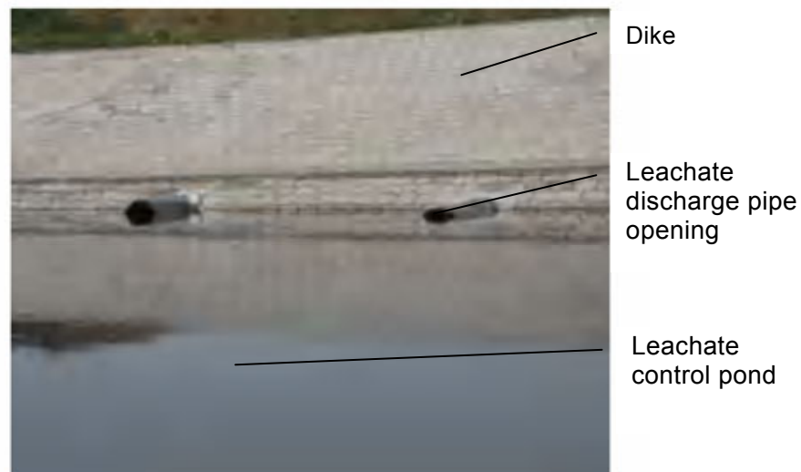
Picture 2-6 Example of leachate discharge pipe opening being submerged
