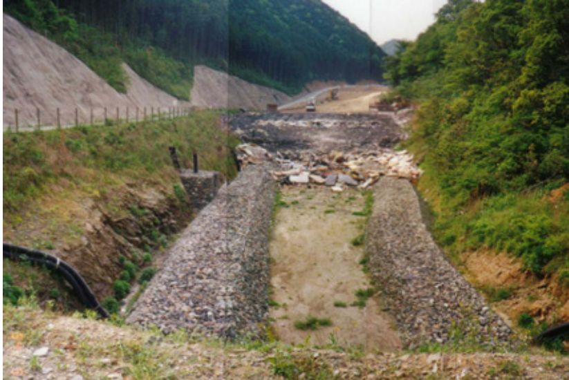
Picture 3-3 Example of landfill of rough waste material in the vicinity of leachate collection discharge pipe
