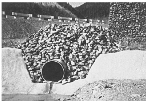
Picture2-16 Example of bottom leachate collection pipe and gas venting pipe
