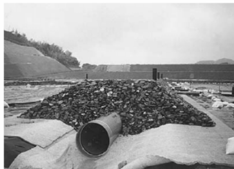
Picture 2-12 Good example of main leachate collection pipe
