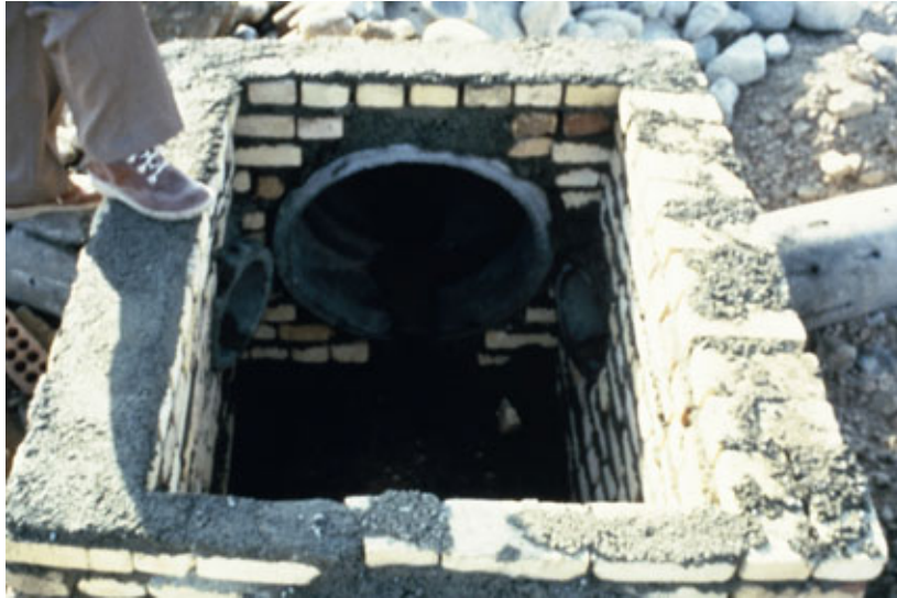
Picture 2-2 Example of using bricks as the leachate collection discharge pipe connection box material
