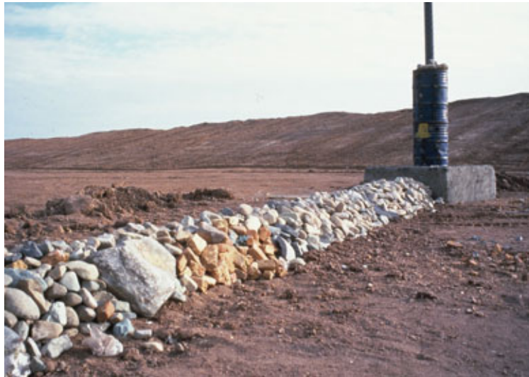
Picture 2-4 Example of using waste barrels as protection material for gas venting pipes
