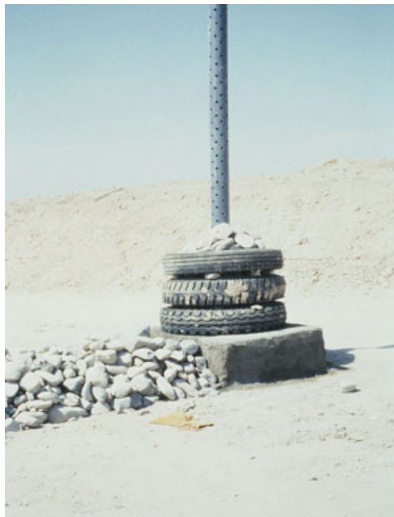
Picture 2-3 Example of using waste tires as protection material for gas venting pipes
