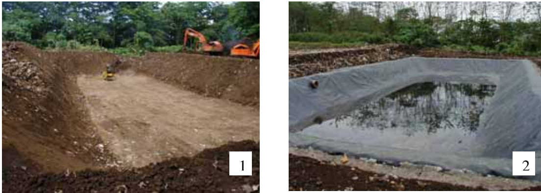
Photo- 20: Leachate Retention Pond
