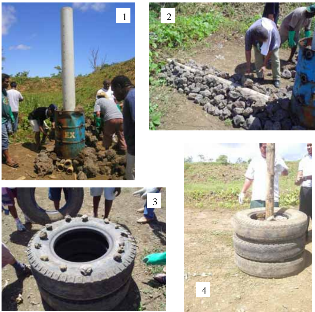
Photo- 25: Application of Used Materials for Leachate/Gas Control Facility
