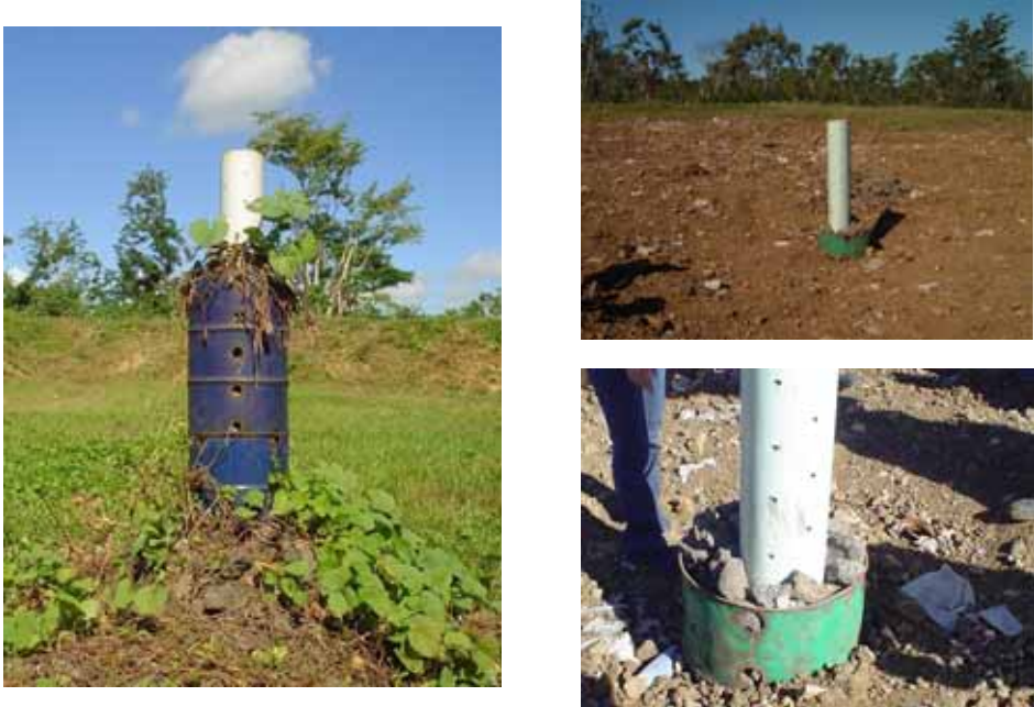
Photo- 24: Vertical Gas Venting Pipes at Landfilled Area
