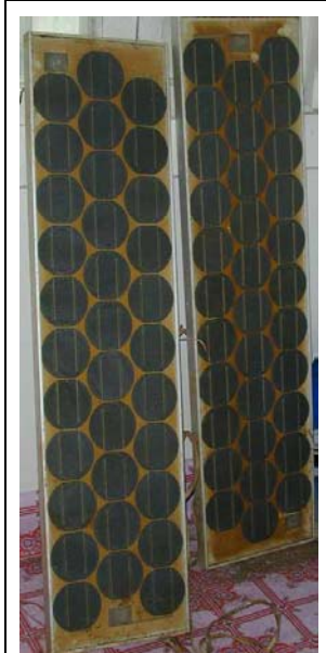
Figure 6-1 - Corroded BP Solar Panels from 1985 Ha'apai projects
